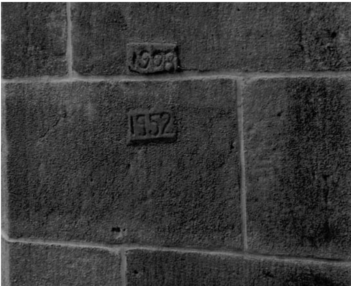
A close-up inspection of the church's walls revealed cement patches showing dates of the last two major repair campaigns — 1908 and 1952.
