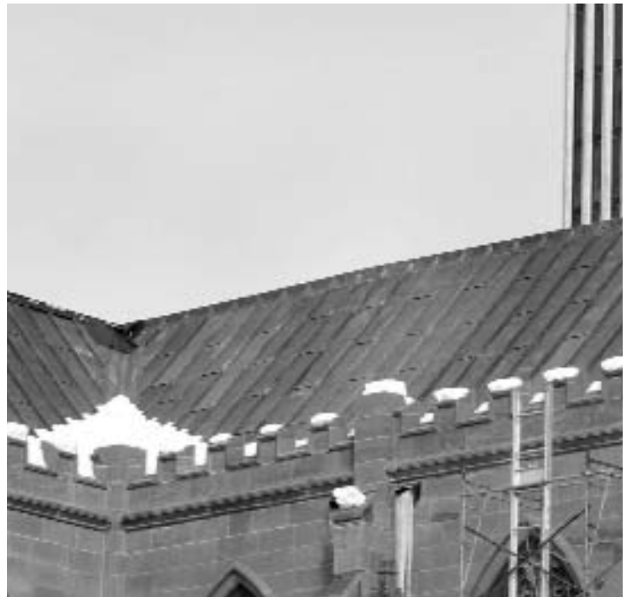
The Cathedral's lead roofing, drainage system, and re-created crenellated parapets were installed in 2002.
