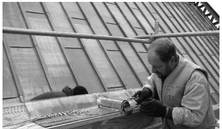
Crews installed the new lead roof with rolled seams at 24-inch intervals.
