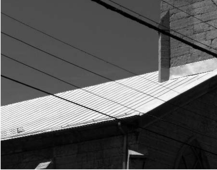
Fair Street Reformed Church in Kingston, NY replaced portions of its terneplate roof with a modern version of the material.
