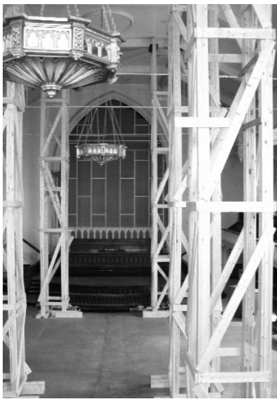
With funding from the Landmarks Conservancy, massive shoring was installed from basement to roof to support failing trusses until repairs are completed.
