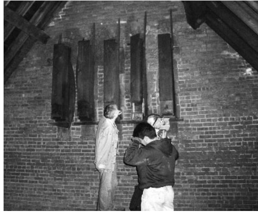
Air baffles that were blocked with debris were cleaned during the restoration.
