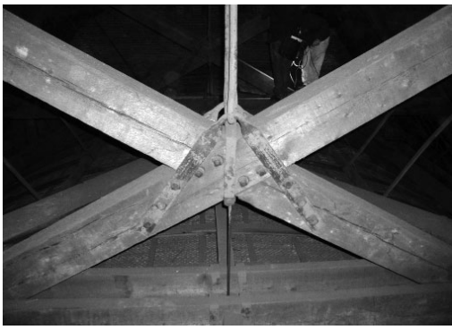
The attic, with its massive wood truss beams, lack safe walkways.
