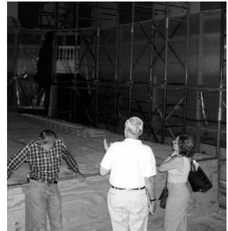
Dave Elligers and Robert Buonvino, president of the New Utrecht Historical Society, inspect shoring at church interior with Ann Friedman of the Conservancy.
