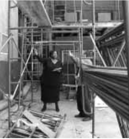
Building conservator Kandace Simmons and Andrzej Kaczmarek of Midtown Restoration discuss masonry restoration at Chambers Memorial Baptist Church.
