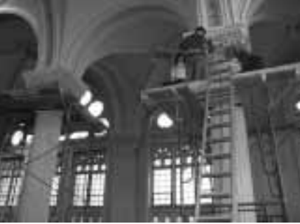
Project architect Kai Woo and consulting engineer Evan Axelrod, of Anchor Consulting, investigate interior column steel and terra cotta at Mt. Morris Ascension Presbyterian Church.
