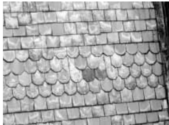
St. James Episcopal Church in the Fordham section of the Bronx deciding to replace their 135-year-old, Pennsylvania slate roof with slate.
